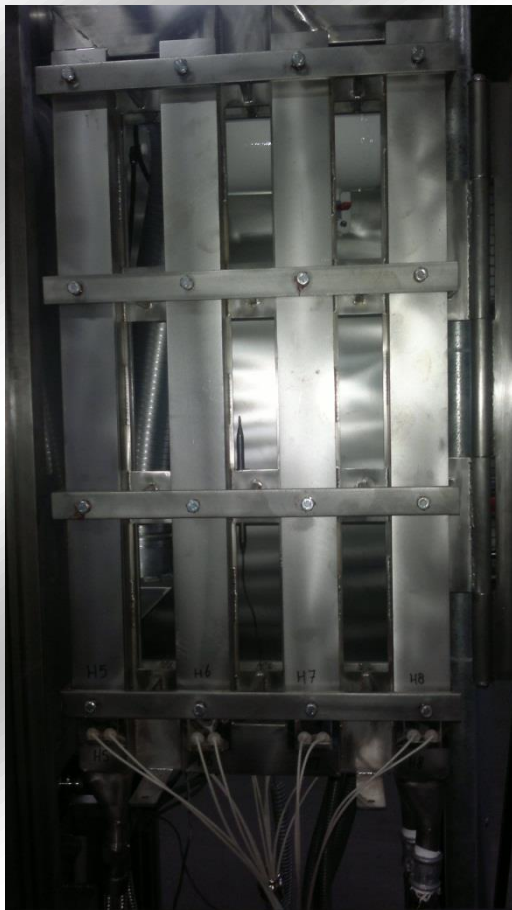
Separate Heat exchanger for Air knives.
