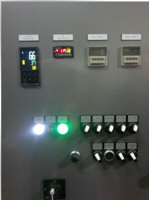
Electrical control panel
